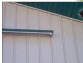
Exterior track cover protects the door system.
